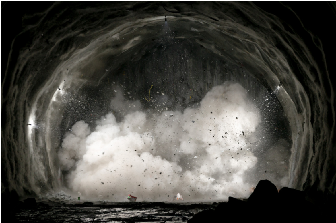
Andrea Botto, "Underground Blast #03", Brenner Base Tunnel, 2020 (courtesy Ghella e Galleria Cartacea).
