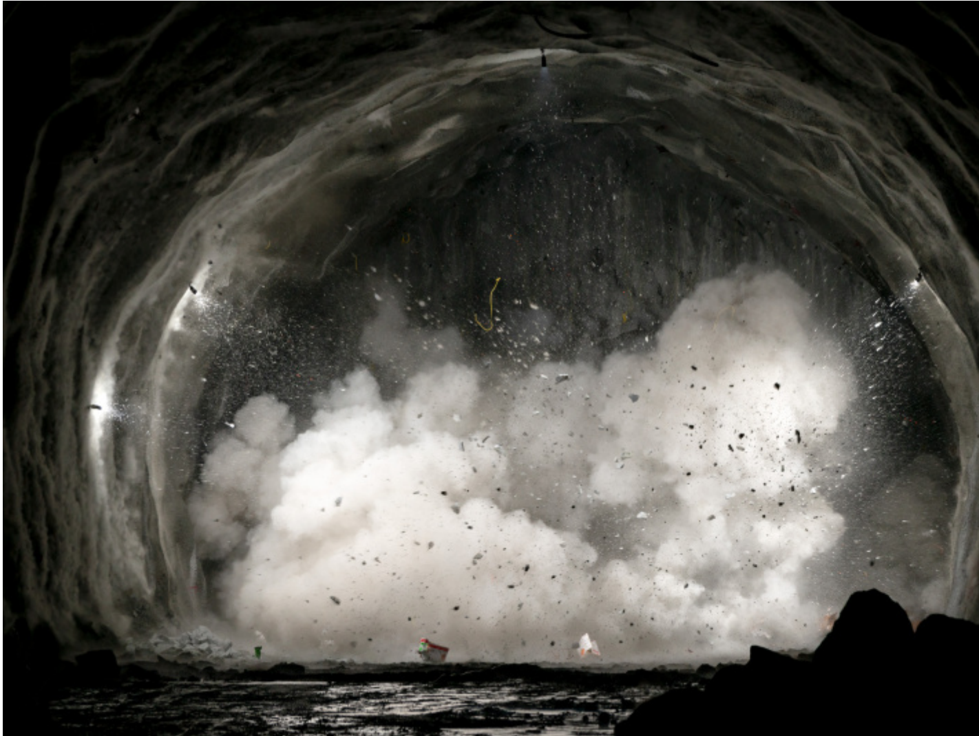
Andrea Botto, “Underground Blast #03”, Brenner Base Tunnel, 2020 (courtesy Ghella e Galleria Cartacea).
